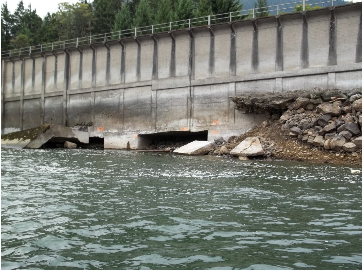
Figure 2 – Photo of 2011 Eroded Area during 2012 Repair
